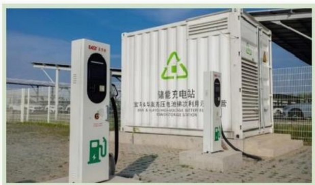
BMW Battery Recycle Power Storage Station
