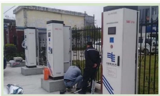
China Southern Power Grid
